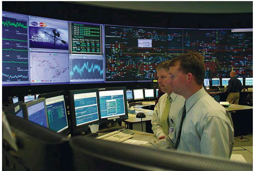
1. The control center of a large organization gets its raw data from sensors in the SCADA system. (Source: All About Circuits)
